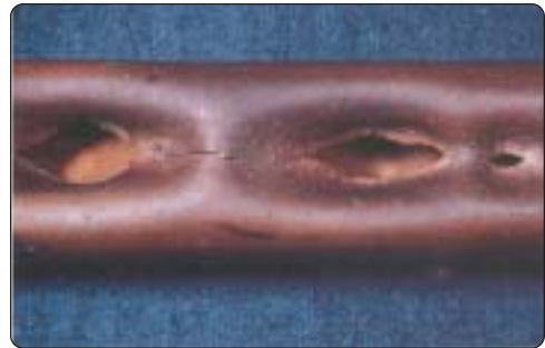
Fig. 2. Tube Damage from Steam Hammer.
